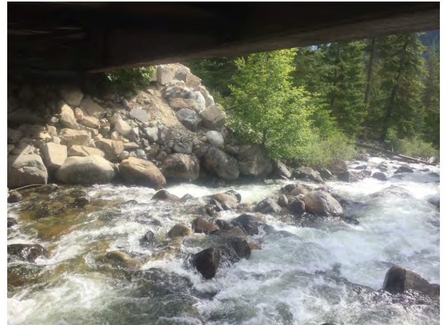
Downstream left bank riprap steep and rounded
